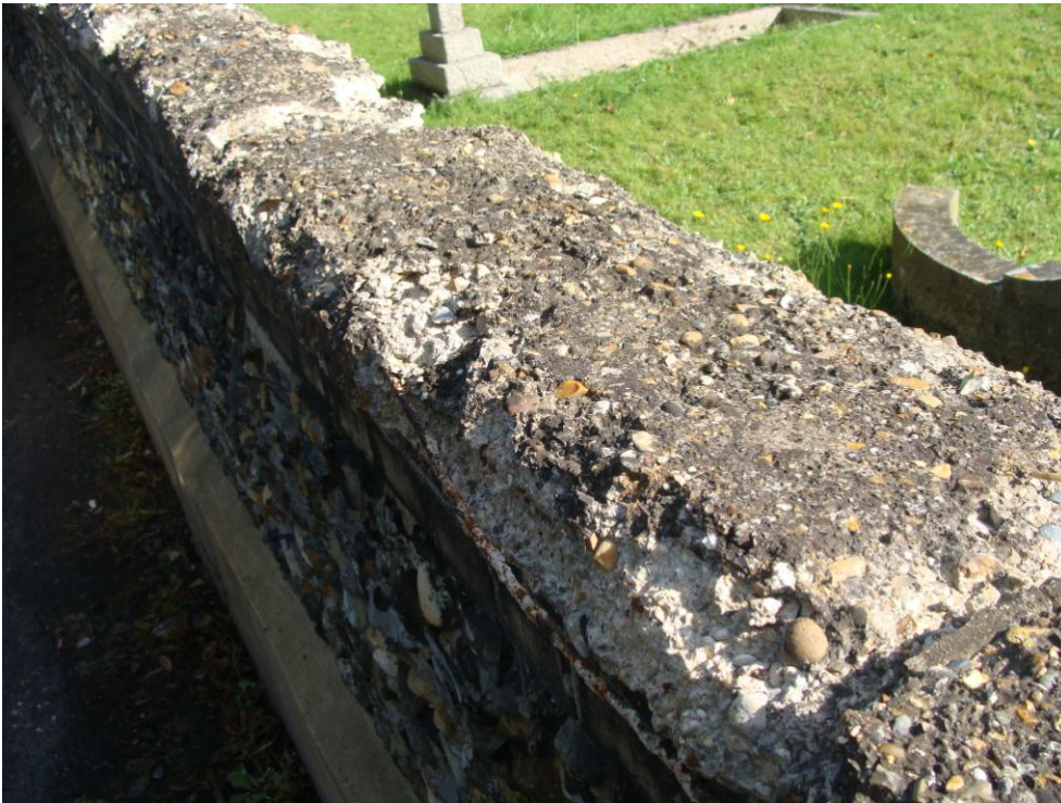
Picture 13 – Concrete capping slabs to church boundary wall in need of replacement.
