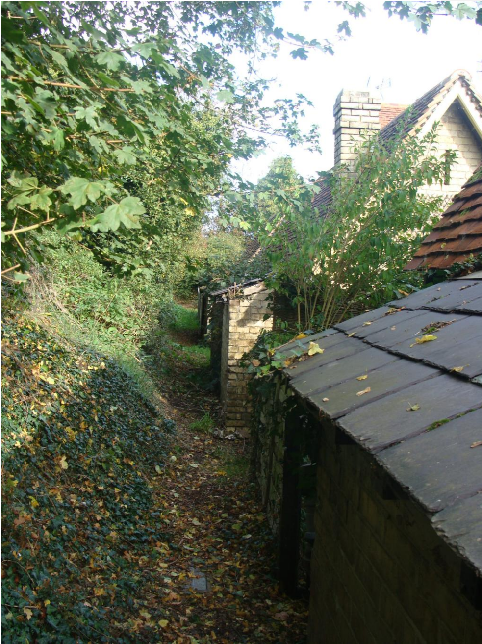
Picture 12 - Outbuildings to nos. 260 - 274 Hertingfordbury Road, that should be retained; particularly important from an historical perspective.
