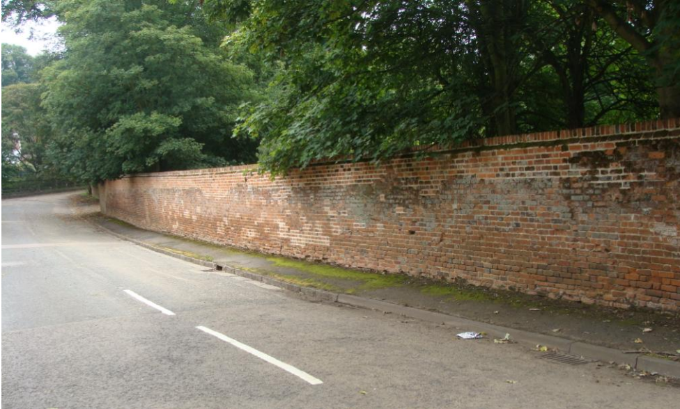
Picture 15 – Western boundary wall to ‘Epcombs’, a prominent and important feature, protected virtue of being within the curtilage of a Listed Building.
