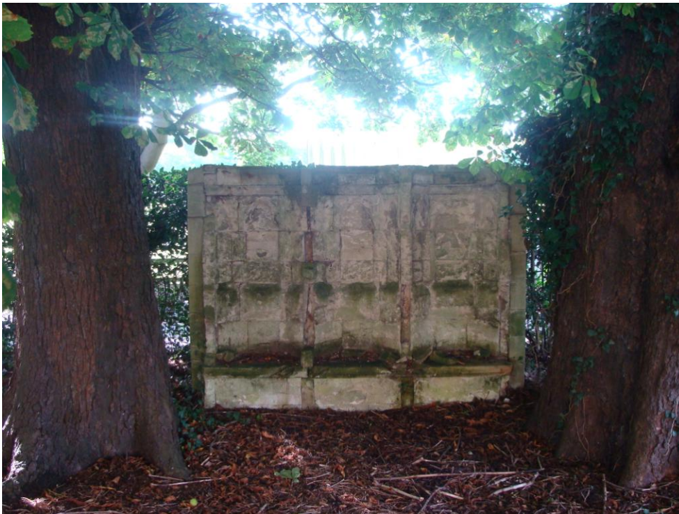
Picture 4 – 14 th century grade II Sedilia removed from church during 19 th century 'restoration', now in need of urgent repairs. Included on the Council's Buildings at Risk Register.
