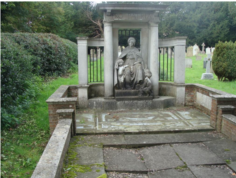
Picture 5 – A fine early 20 th century memorial to Pauline Payne Whitney Paget, in need of repair, listed grade II.
